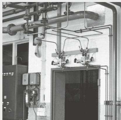
Monitoring for grease and oil ingress in two separate condensate return lines
